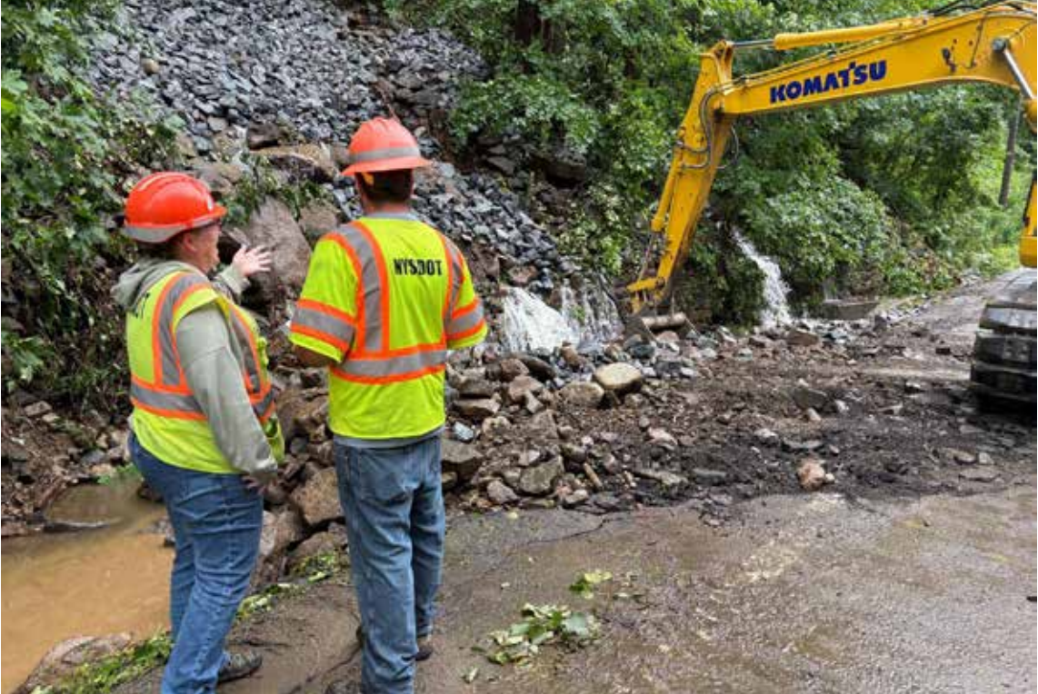
On July 30, NYSDOT staff were on site on Route 9 in Fishkill surveying the damage, evaluating repairs, and planning the safest, fastest path to restoring the roadway. Photo Credit: NYSDOT
