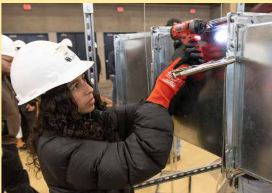
Sheetmetal Workers L.U. 38 of Brewster, NY.
