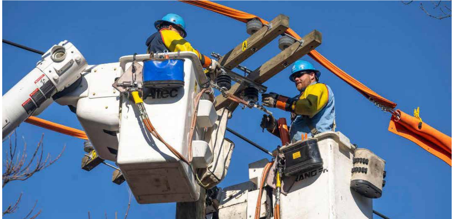
The proposed electric and gas rate hikes will support economic growth and development in New York City and Westchester County by investing more than $21 billion over three years (2026-2028) to build new infrastructure. Pictured are Con Edison Electric operations workers on the job. PHOTO COURTESY OF CON EDISON
