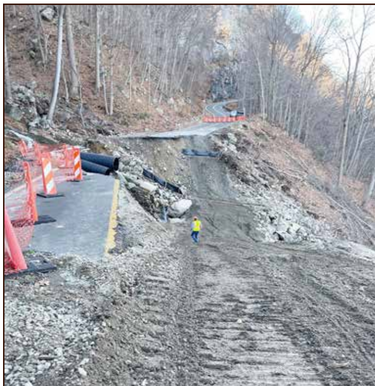
A section of Route 218 in the Town of Highlands, NY in Orange County suffered extensive storm damage in July 2023.
