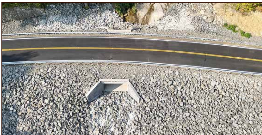
The extreme storm damage required a full rebuild of the downhill slope with more than 35,000 tons of recycled, light, medium and heavy stone fill used in the reconstruction.
