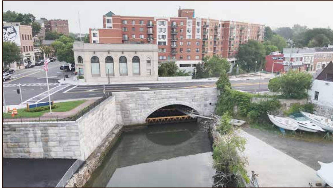
The new bridge over the Mamaroneck River structure was constructed off trusses that spanned the entire width of the river under the existing bridge.
