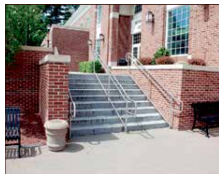
Iona College Student Union in New Rochelle, NY, where the company performed masonry work for Darland Associates, Inc.
