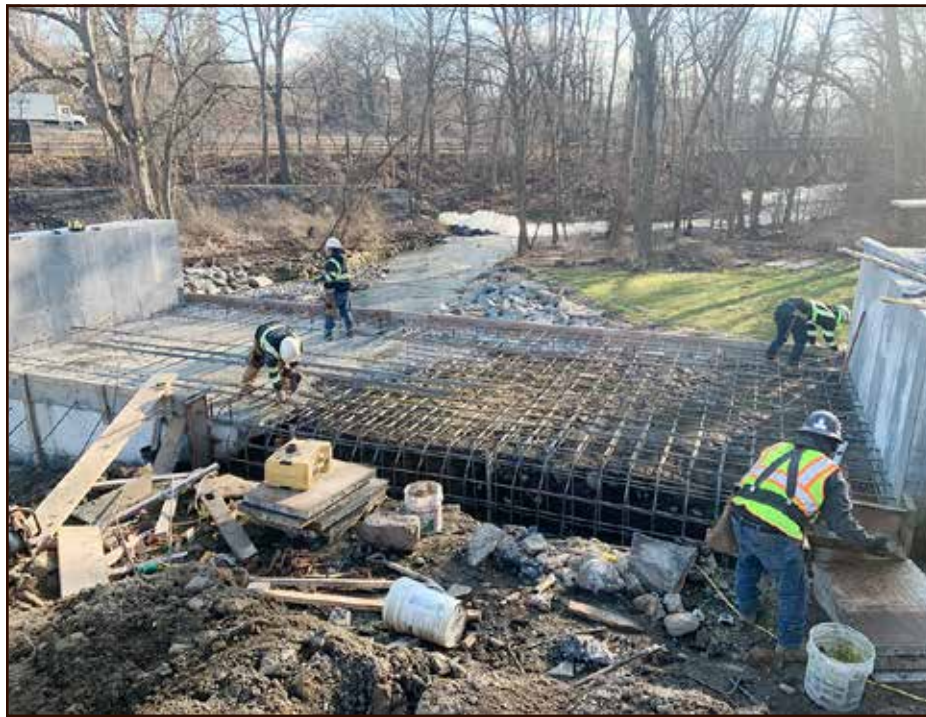
Crews setting rebar in mid January on the Woodlands Lake Dam Removal capital improvement project in Westchester. With the dam removed and a new bridge being built, the project diverts water into a new river channel flowing parallel to the trailway in the Town of Irvington.
