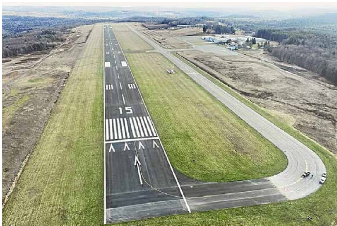
Construction work has already begun on the $24-million project to build a new terminal at the Sullivan County Airport. The project will be performed under a Project Labor Agreement. Bids were due to be awarded this month.
