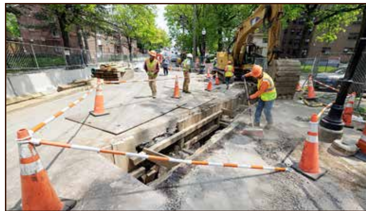
Mount Vernon is tapping $9 million in Clean Water Infrastructure Act funds for engineering, design and construction work associated with the Third Street Sewer Project.
