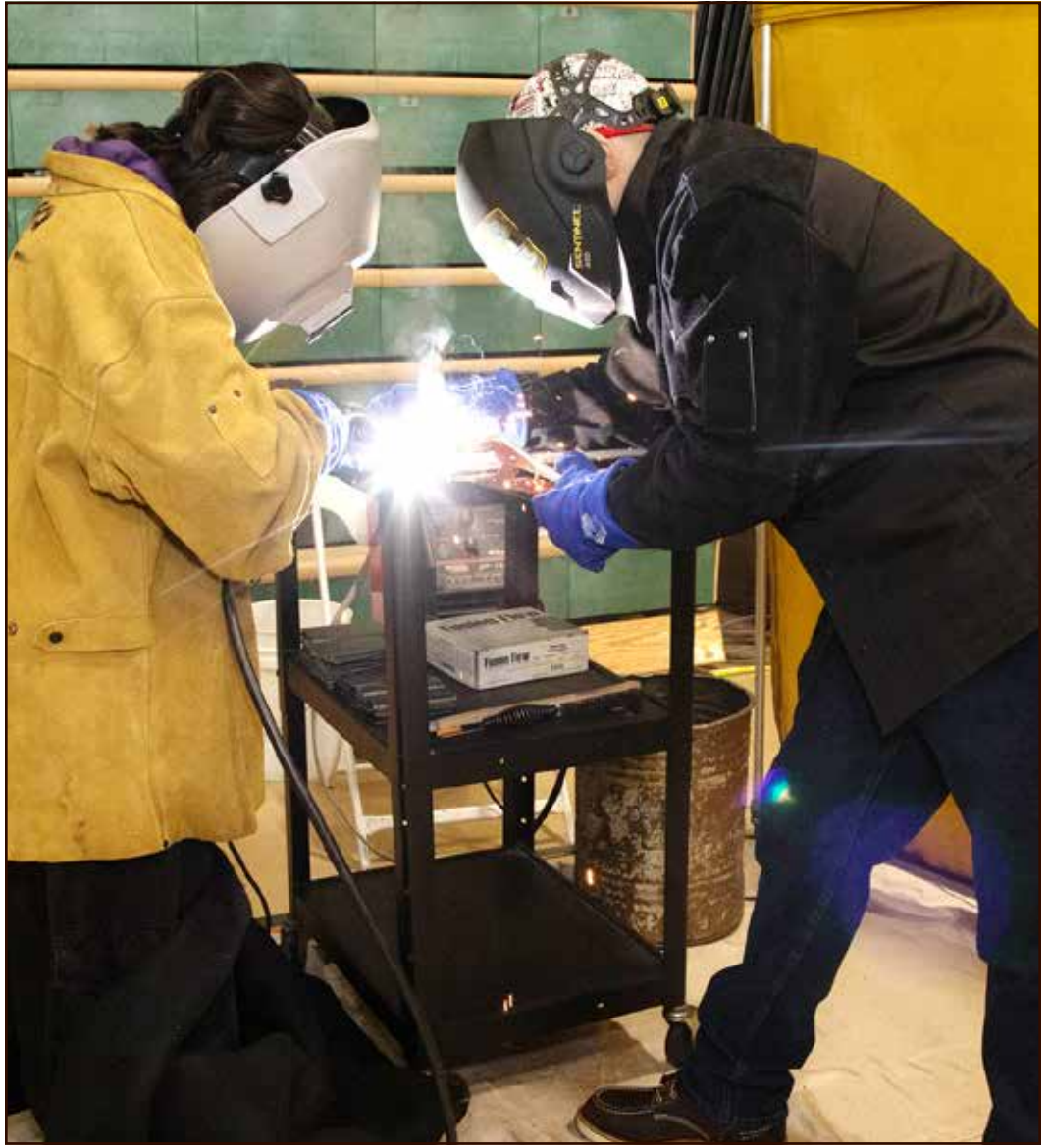
Welding always attracts attention. Ironworkers L.U. 417 and 580 were among the 17 trade locals that attended the apprenticeship career exposition.
